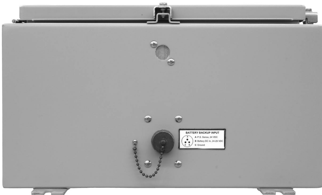
Figure 2: Bottom view of cabinet enclosure.
